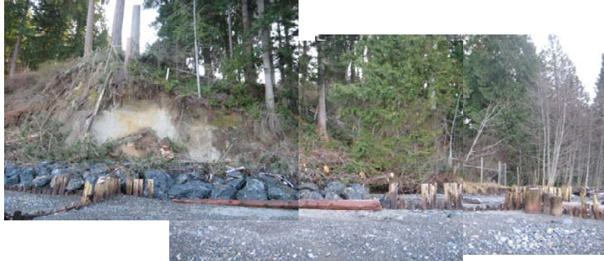
Figure 3: View of Shoreline Showing Remnants of Cedar Seawall
