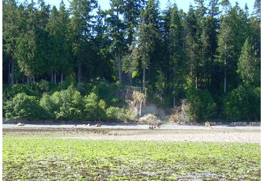
Figure 2 Photo of the Milner Property, looking westward across the intertidal zone. While most of the cliff is covered with trees and shrubs, the bare portion in the centre has recently failed.
