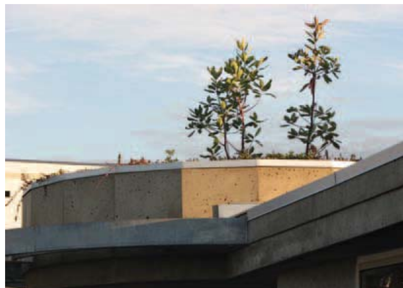
Top photo: Green roof on garden shed, Michigan Street Community Garden. Bottom photo: Green roof on Burnside-Gorge Community Centre. PHOTOS: CAROLYN MASSON
