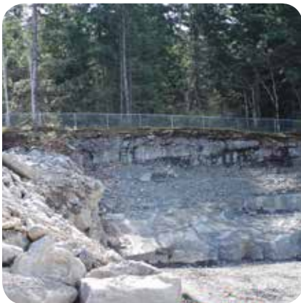
Seepage zone intersected in rock cut is draining the ephemeral pool in an adjacent GOE at Mt. Tzuhalem Ecological Reserve. Designing the development with minimal blasting would have prevented this problem. Photo: D. Polster
