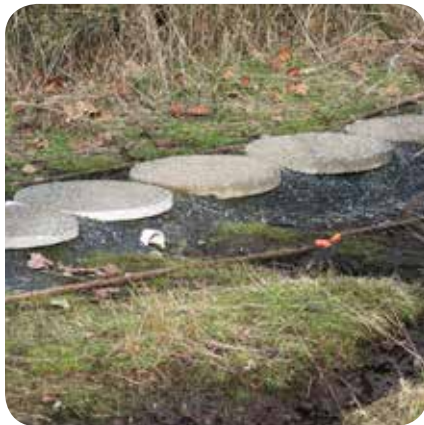
Pipe installed to allow water to flow through a trail at Mill Hill Regional Park. Photo: J. Miskelly
