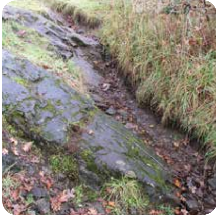
Gully in a hiking trail caused by soil erosion at Mill Hill Regional Park. Photo: C. Maslovat
