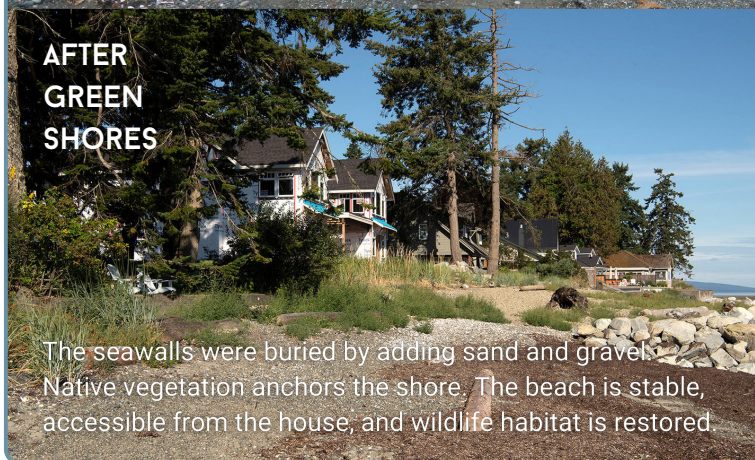
Significant erosion and drop in beach height due to reflected wave energy scouring the foreshore. Seawalls are overtopped during storms, flooding the property.
