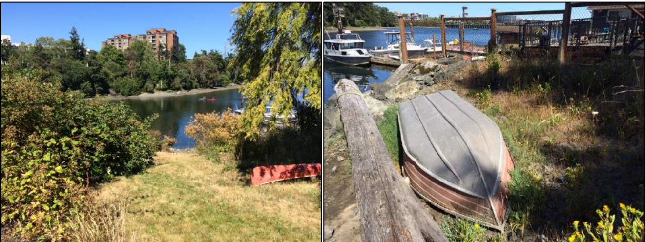
V02 – Ongoing maintenance required: invasive species removal, additional native planting, and alternative boat location.
