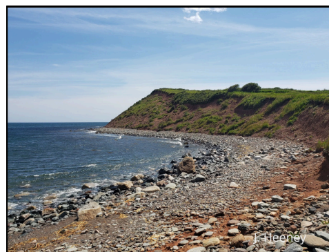
A natural, cobble shoreline backed by an eroding bluff in Nova Scotia.
