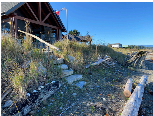
The Admiral Tryon Boulevard site in BC is an example of a GSH hybrid design Reinforcing project using a buried revetment to protect against high wave energy and erosion from high tides and storms (8). Photo above shows site 3 years after Green Shores certification.
